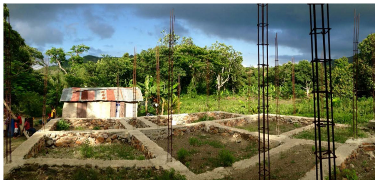
Fig. 5 New home construction in Haiti by a worker allowed to work in the USA. In the foreground is the foundation for the new home of a worker allowed to work in the USA in 2015, under construction in 2016 for his family of seven. In the background is his current two-room home. This was taken on May 22, 2016 in Milot, Nord, by Hannah Postel
